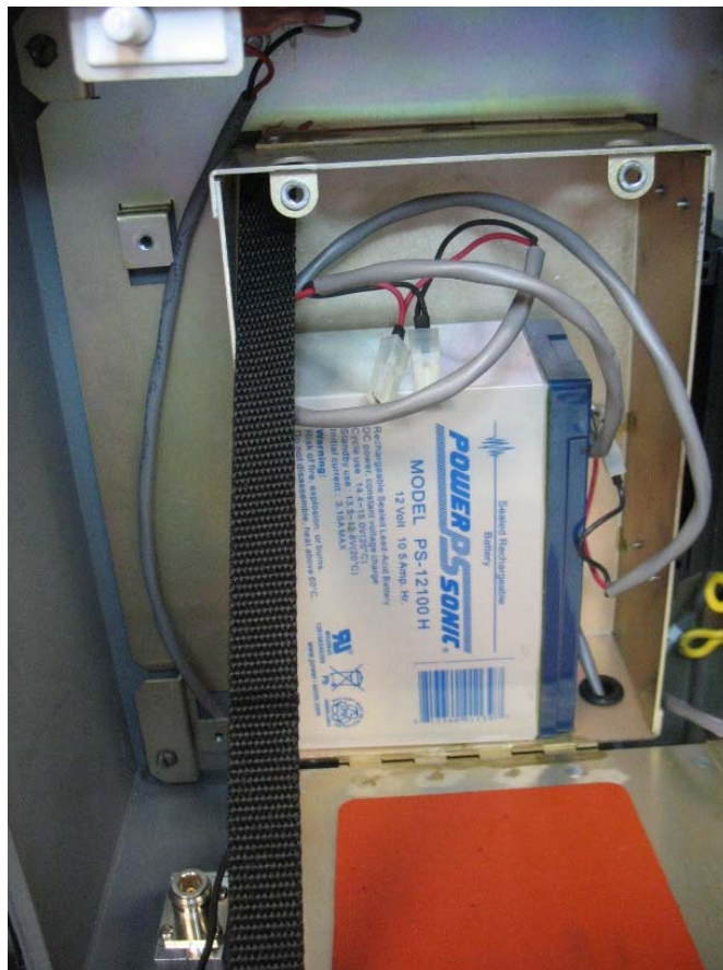
Figure 2-30: Battery Pack Attached to Compartment
