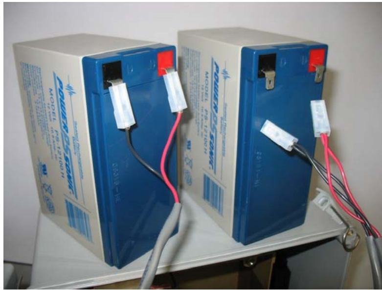
Figure 5-11: Old Battery (left) and New Battery (right) Sit on Enclosure
