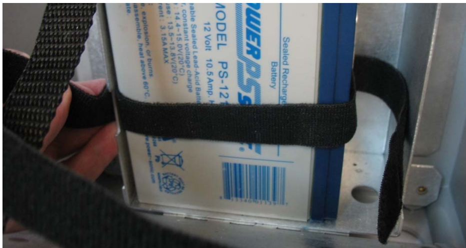
Figure 2-28: Battery Pack Attached to Compartment
