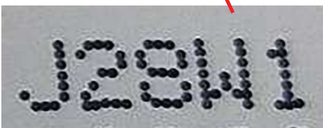
Location: side of circuit breaker.
