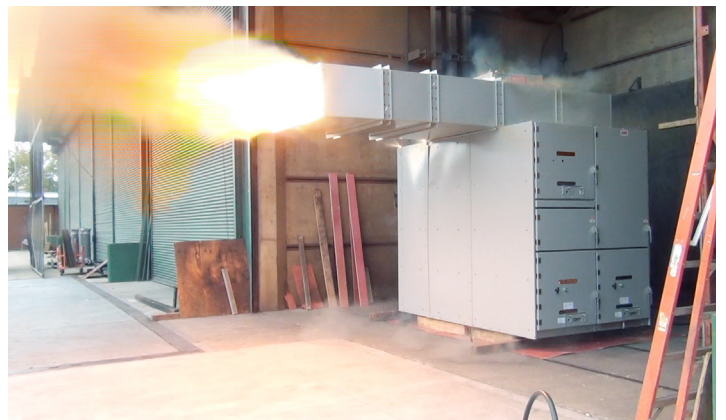
Arc-resistant switchgear 63 kA interruption at KEMA Test Lab
