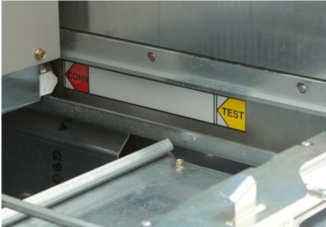
Figure 24: Circuit breaker in CONNECTED position
