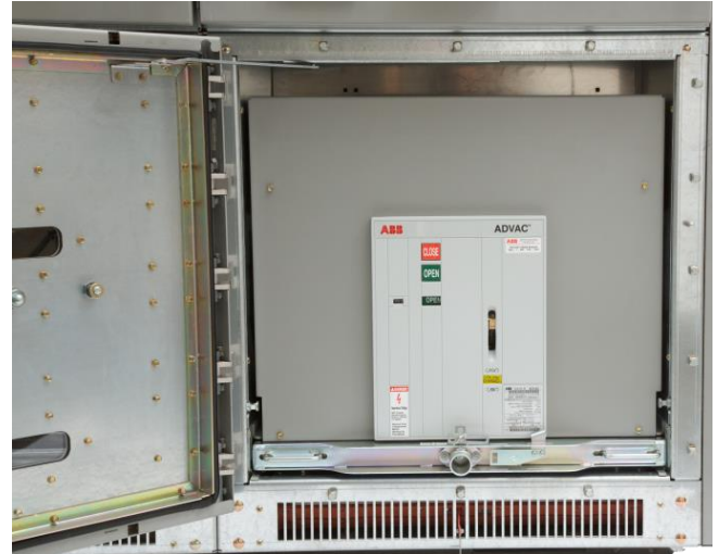
Figure 20: Circuit breaker in DISCONNECT position
