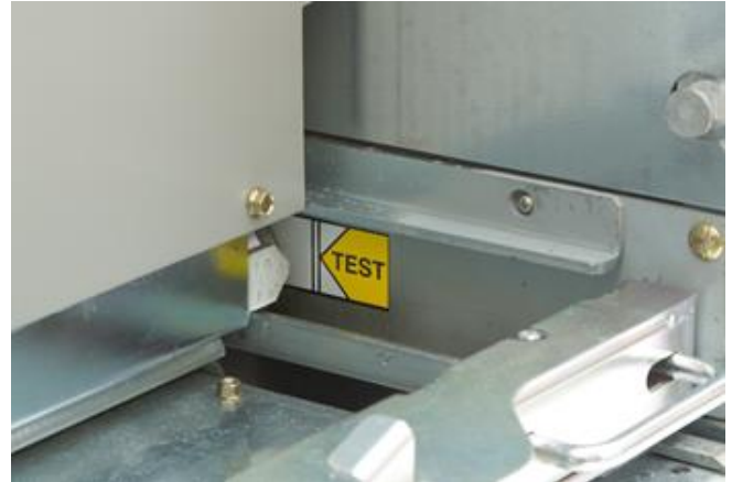
Figure 23: Circuit breaker in TEST position
