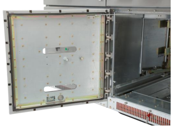
Figure 12: Breaker Cell door open
